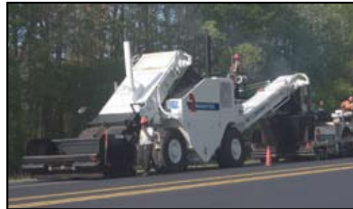
The Shuttle Buggy MTV continues to feed the paver while trucks are on their way. A 25-ton (22.7 metric tons) surge bin makes it possible.
